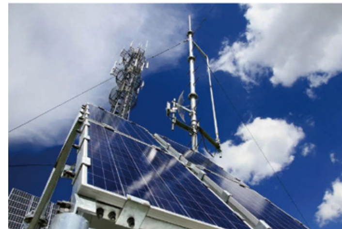
Communication Base Station
