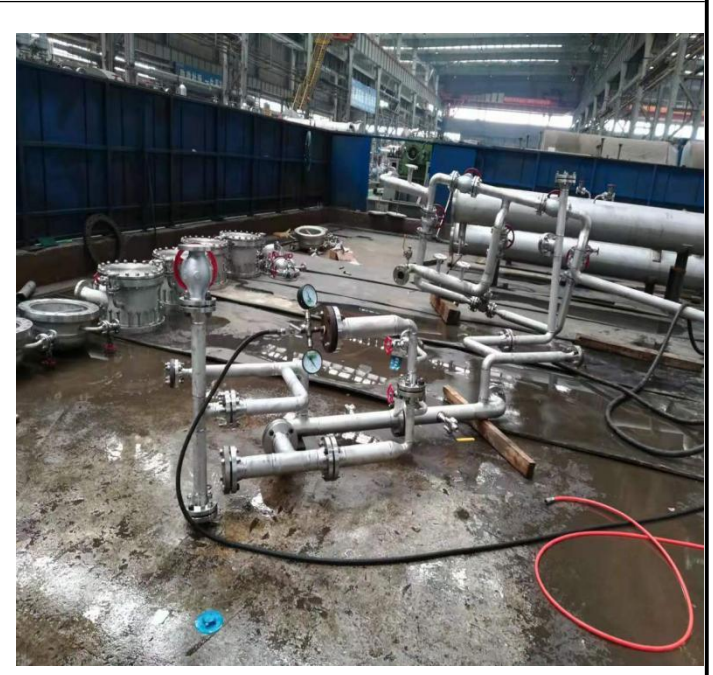
4. The hydrostatic pressure test for piping of Regeneration Gas Compressor of product no ***
