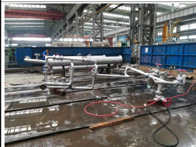
7.The hydrostatic pressure test for piping of Regeneration Gas Compressor of product no ***
