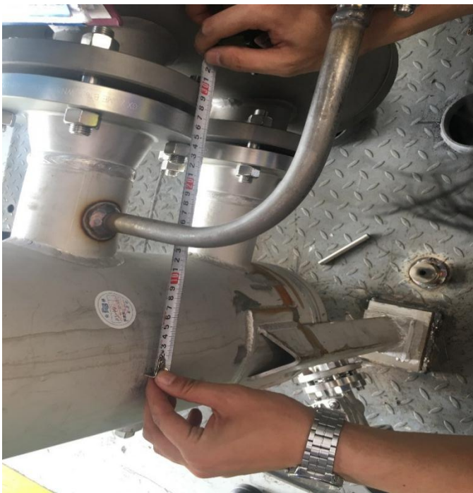
13. Measurement of flange dimension from shell to change over valve (product no ***)
