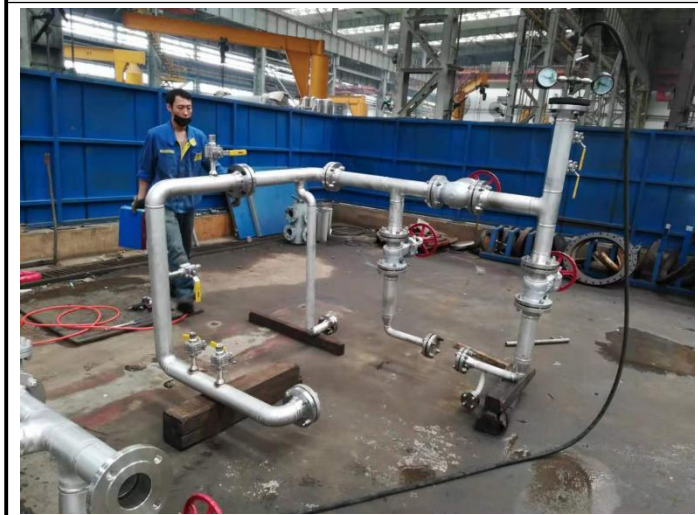
1. The hydrostatic pressure test for piping of Regeneration Gas Compressor of product no ***
