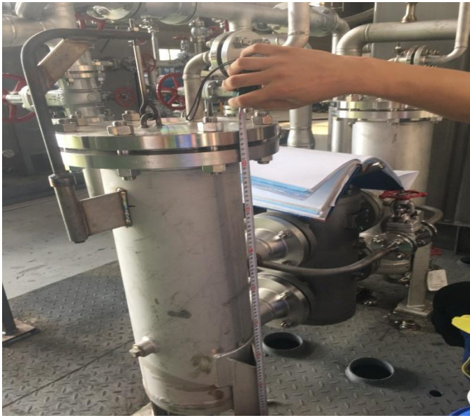
11. Measure the shell height of oil filter for Regeneration Gas Compressor of product no ***
